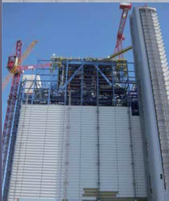
E-on power station, near Rotterdam, The Netherland
